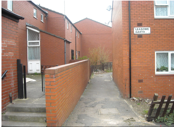
Entrance to footpath from Leasowe Garth end – criminal damage to fence next to footpath
