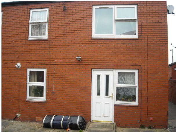
Insecured bedroom window at rear of property and Euro Profile locks that are susceptible to tampering
