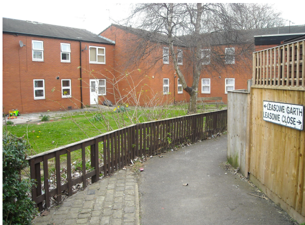
Access to courtyard from Leasowe Close – damage to picket fence
